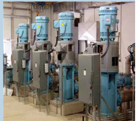
Ruhrpumpen Water Pumps City of Brantford (Ontario, Canada)
