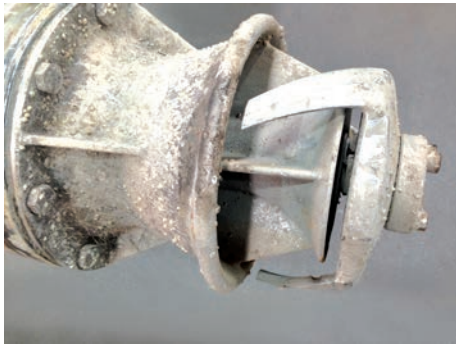
Original damaged part
